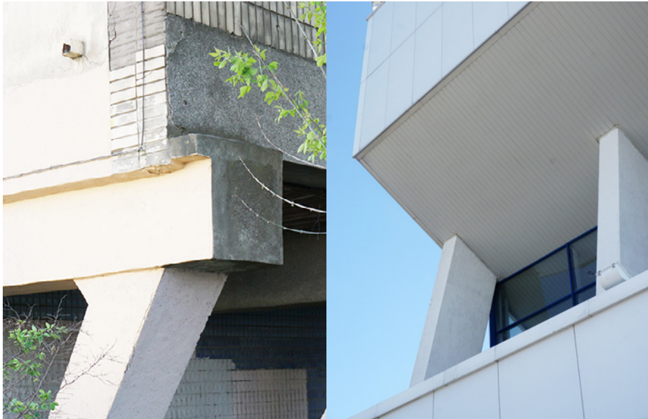
Figure 11: This building corner offers a retrospective of Soviet Modernist coatings: concrete construction is covered by granite sand and light-yellow matt ceramic tiles, both partially missing; several shades of paint on the balcony screen of, probably, asbestos; blue glazed ceramic tiles decorating the street-level-wall; recent overpainting with light colors. Figure 12: Aluminium-coated panels. Source: Author
