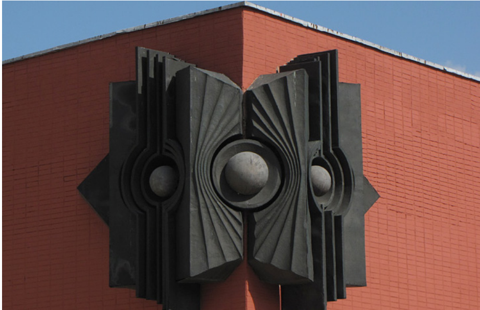
Figure 7: During reconstruction works on the cinema "Electron" (serial project, built in 1981) missing tiles, mimicking brick, were replaced by an imitation themselves: the peeled off areas (on the right of the Electron-sculpture) were covered with plaster, onto which a tile pattern was marked. Source: dariuss, https://dariuss.livejournal.com/509940.html
